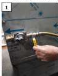
1 GAS VALVE IS CLOSED
